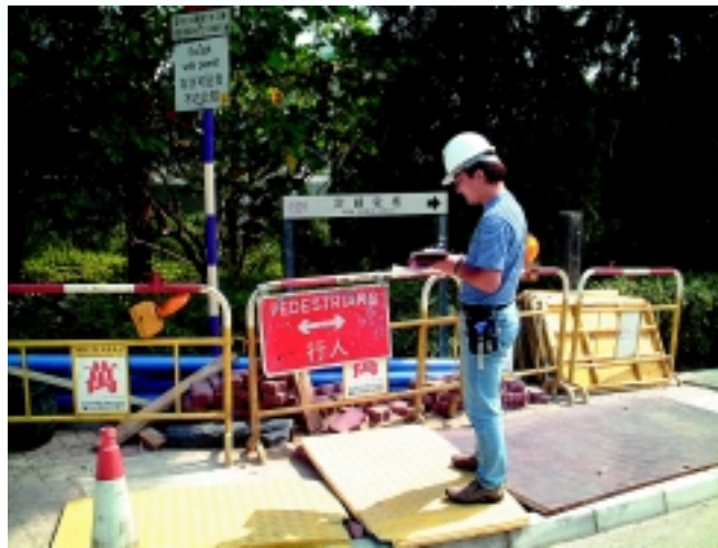
The staff of USEO regularly inspects the housekeeping and safety and environmental compliance of construction sites.
