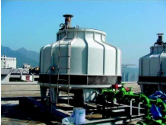
The air-cooled chiller at the Pi Ch'u Building was replaced by a water-cooled chiller.
