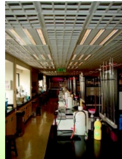
Energy saving T5 Fluorescent Tubes are adopted in the laboratory in the retrofit programme.
