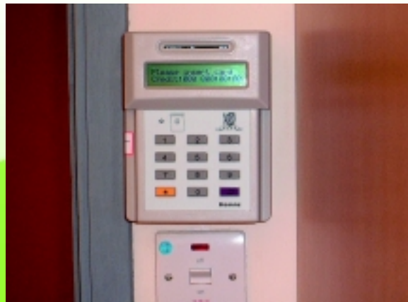
Electricity controller with timer is used in student hostels. 學生宿舍電力控制器設有定時開關。
