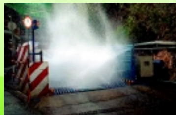
Vehicle washing pool was set up at the entrance of construction sites to clean up the dust.
