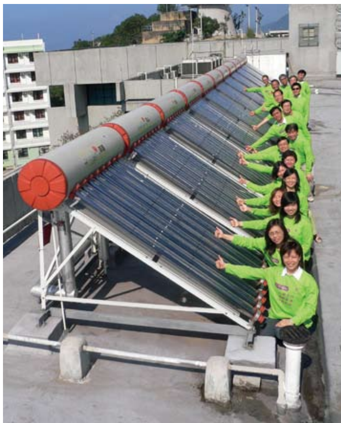
CUHK is the first university in Hong Kong to instal solar-powered water heaters in student hostels
