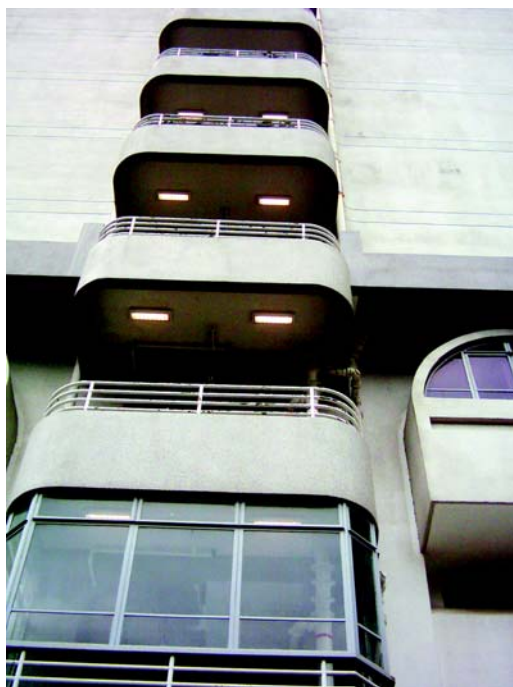
T5 14W Energy Saving Lamp in staircase of BMSB 基本醫學大樓梯間的T5 14W省電螢光燈
