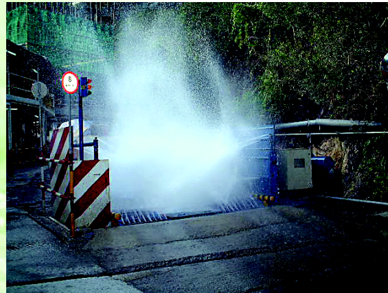
Vehicle washing pool was set up at the entrance of construction sites to clean up the dust.
