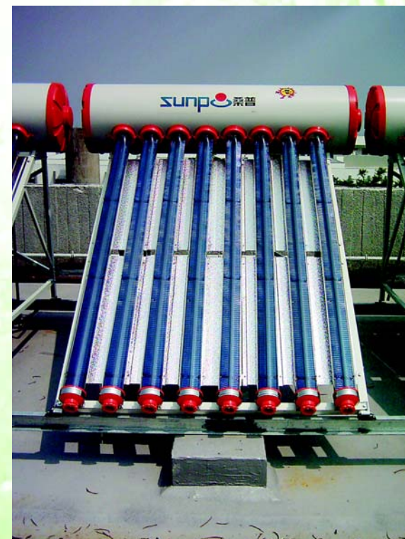
Solar Collectors in Cheung Cheuk Shan Amenities Building 張祝珊師生康樂大樓的太陽能收集器
